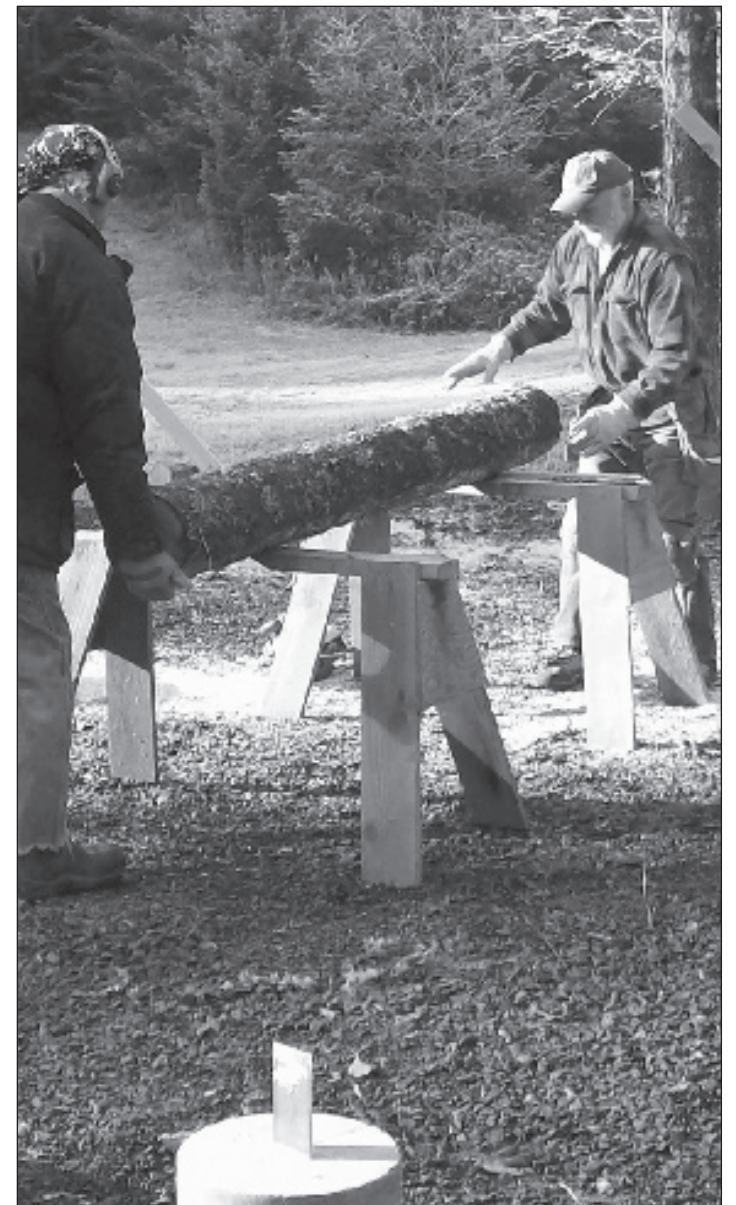
Tom Bauman, left, and Lee Holly work on cutting and fitting poles for the volunteer shelter on a cold and frosty winter morning.
